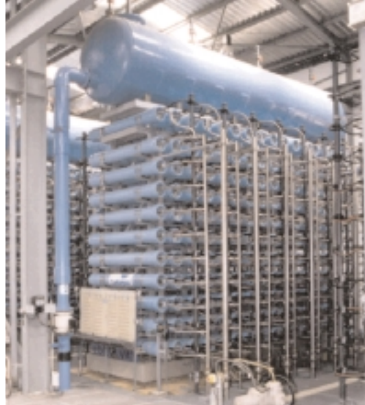
Reverse osmosis membranes
