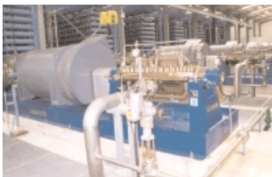
High pressure pumps
