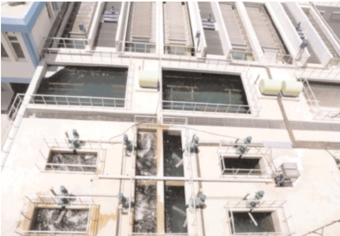
General view of flocculation and sedimentation tanks
